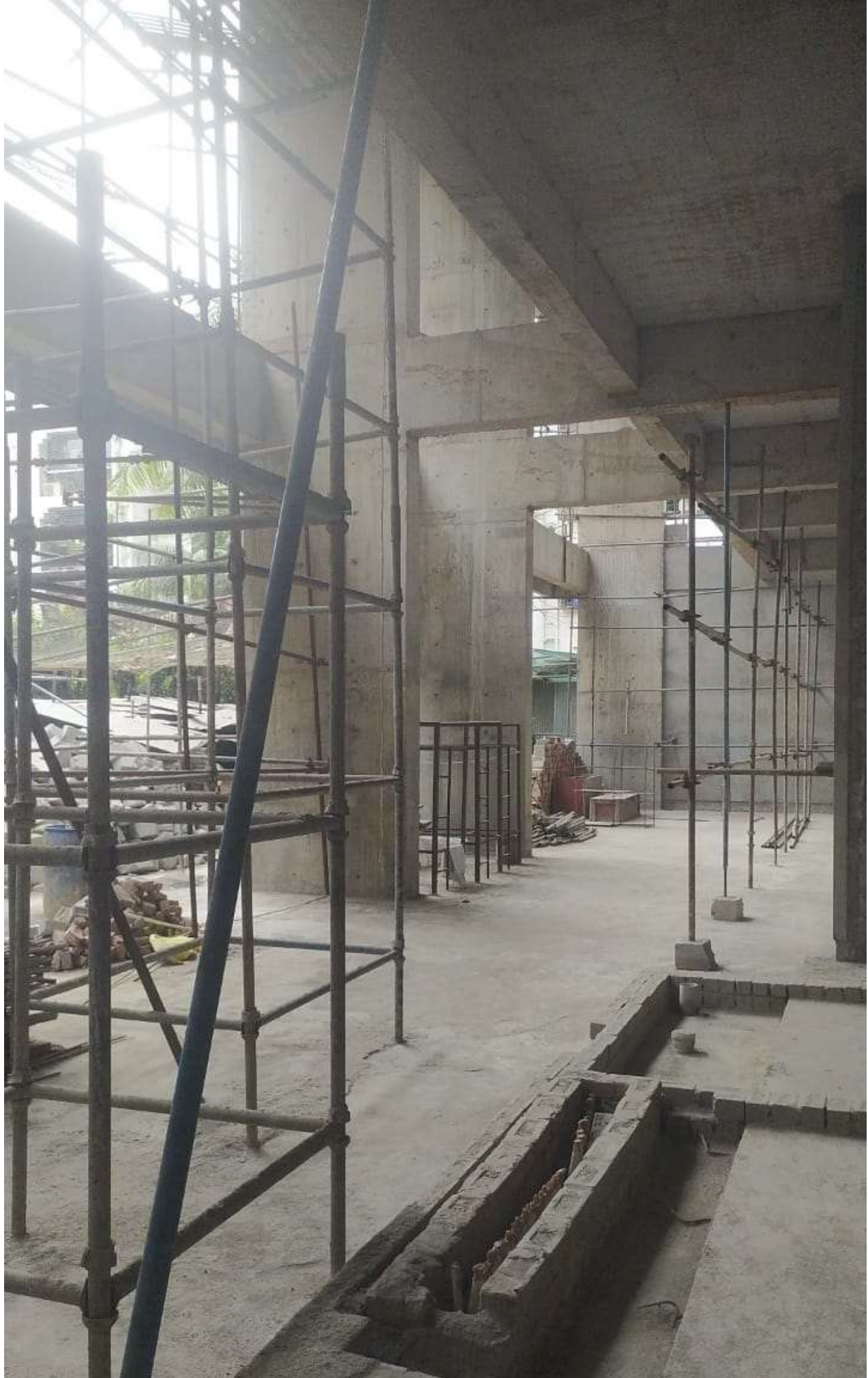
Ground floor South side car parking and electric room
